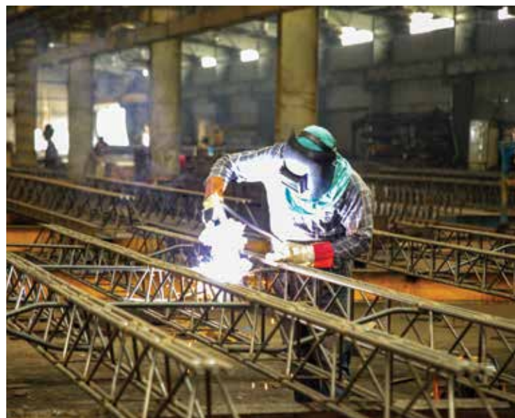
▲ With most of the work done in-house, it's easier to meet quality standards.
